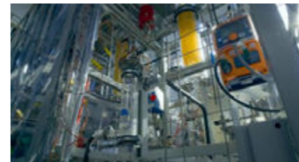
View of CO2 capture plant at CERTH's PSDI Lab
